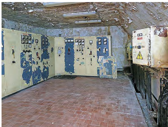
The Soviet-era facilities control room on the bottom floor of Zeppelin/Ranet. Photo Clive Penfold
